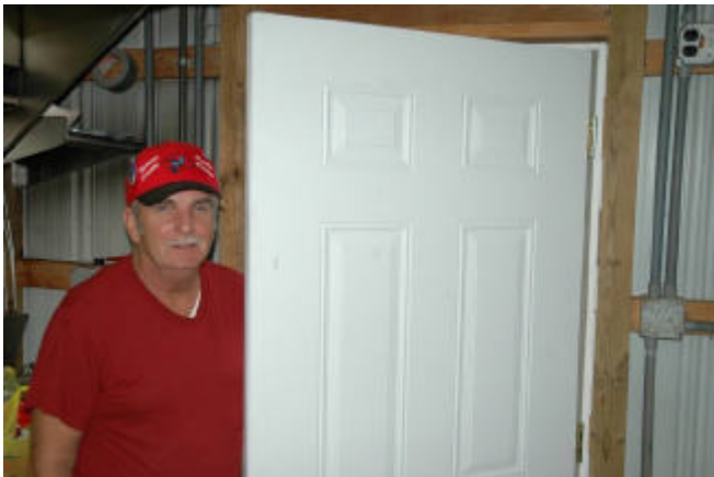
Master handyman Rich Green installed a new six-panel security door on the kitchen.
